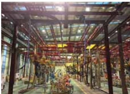
Bus Bar Track System (Car welding line)
