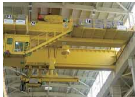
Steam Turbine Over Head Crane(120Ton)
