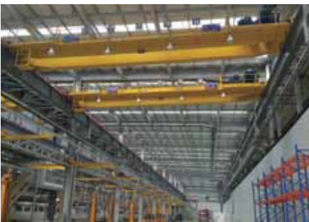
Over Head Crane
