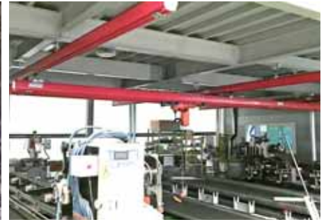
Bus Bar Track System (Welding shop)
