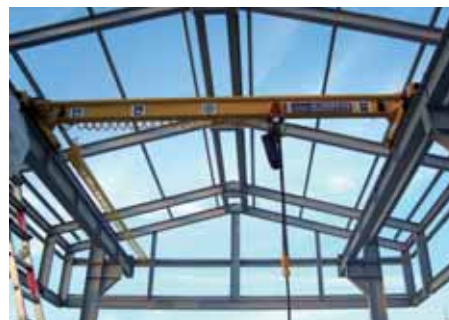
Air type Over Head Crane
