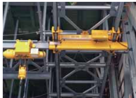
Pulverizer Maintenance Crane (Suspension type 40Ton)
